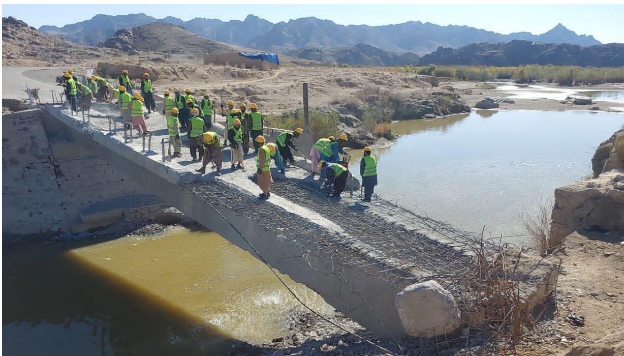
Photo 1. The collapse of Dahla Bridge, Shah Wali Kot District of Kandahar Province, September 15, 2022.
